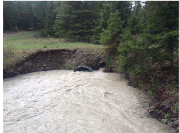
Figure 40. Undersized culvert during spring runoff.
